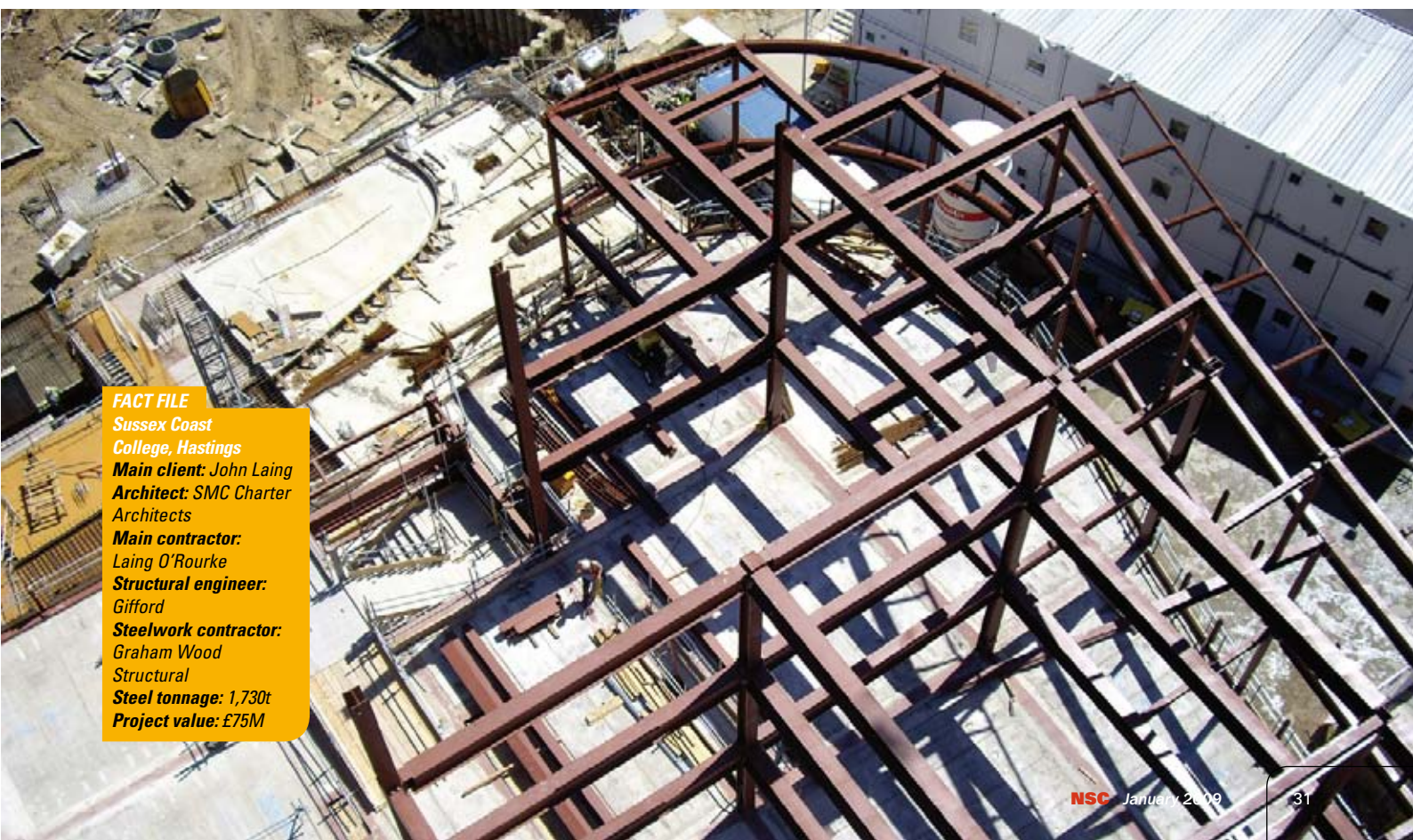
Below: Shallow heavy beams were required to facilitate the installation of the long TermoDeck planks.
